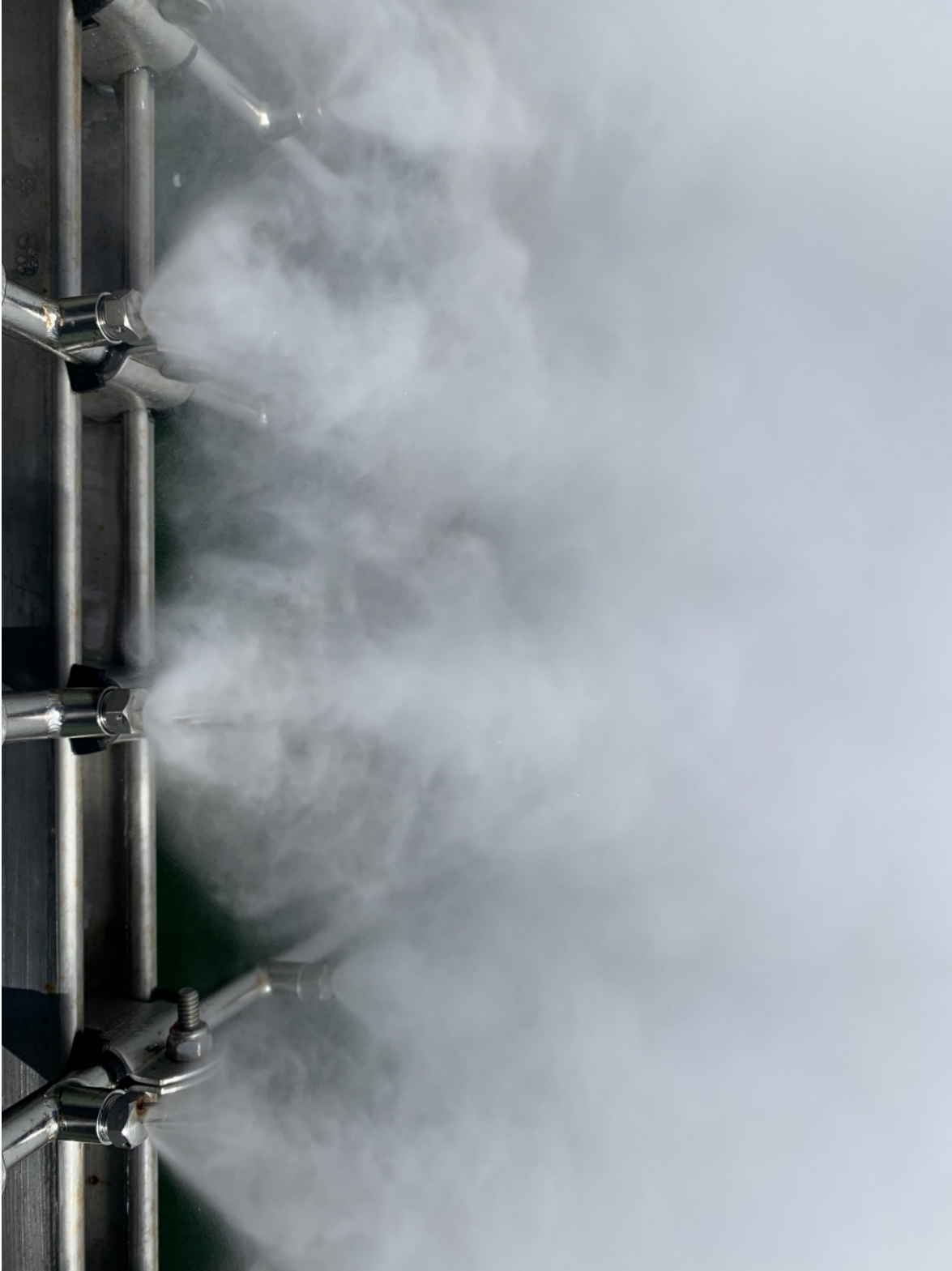
Figure 27: Close up of fogging nozzles during operation on the Great Barrier Reef, 2023.
