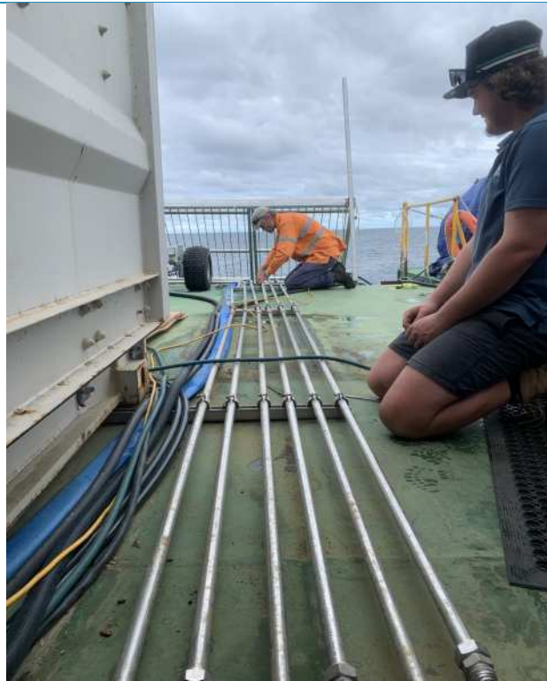
Figure 5: Laying the water delivery pipes for the fogging system prior to field experiments on the Great Barrier Reef, 2023.
