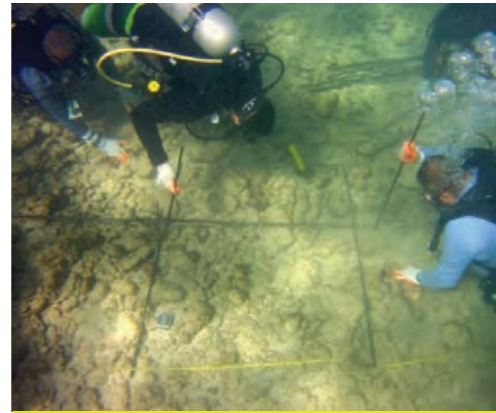
Figure 53. Divers inserting rebar stakes into the substrate to build the supporting framework. Source: Sea Ventures MRU
