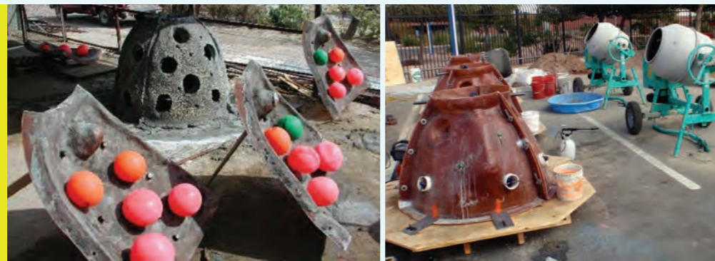
Figure 142. Construction of Reef Balls. Source: Reef Ball Foundation ( www.reefball.org ). Retrieved from https://www.reefball.org/album/index.html
