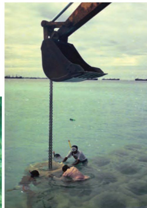
Figure 134. Large 1 m 3 SHED block (hollow concrete cube) being lowered into position on the reef-flat at Galu Falhu, Maldives. Source: Alasdair Edwards
